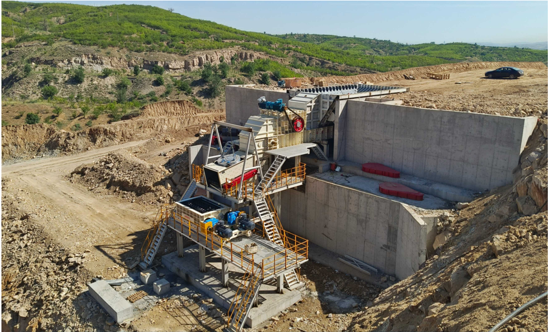
S15 Pro 3/06/21 09:21 1800TPH/SET COAL CRUSHING & SCREENING PLANT/RAW COAL/CHINA
